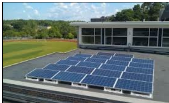
Figure 4 Fairfield has installed roof-top solar panels at several schools in Town, saving on energy costs
